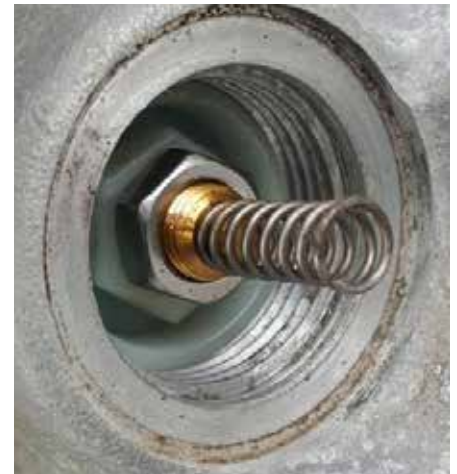
Figure 6. Corrosion found in the test tap after removing the transformer from service
