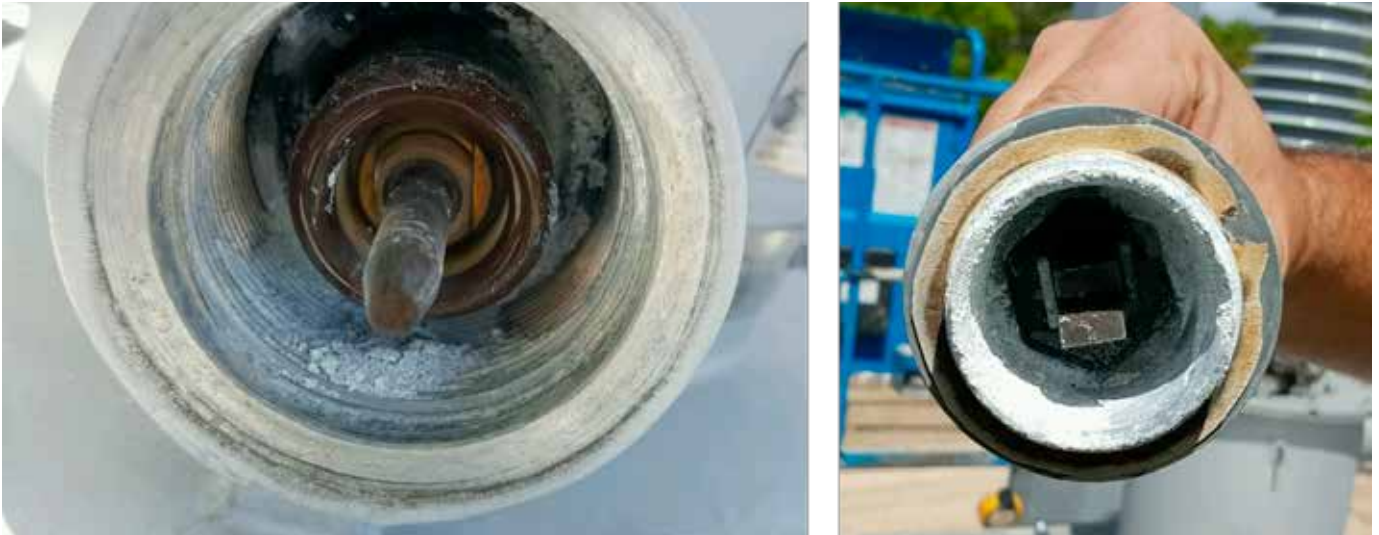
Figure 4. Bushing test tap with moisture ingress due to an improper sealing gasket
